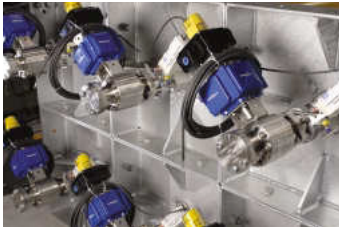
Electro-pneumatic actuated valve assembly.
