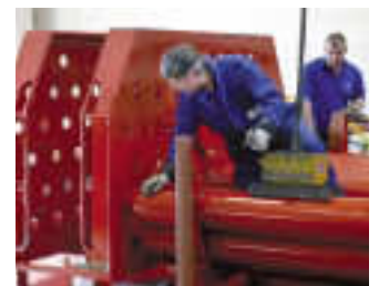
Refitting hydrogen cylinders into a bulkhead of a road trailer unit after refurbishment.
