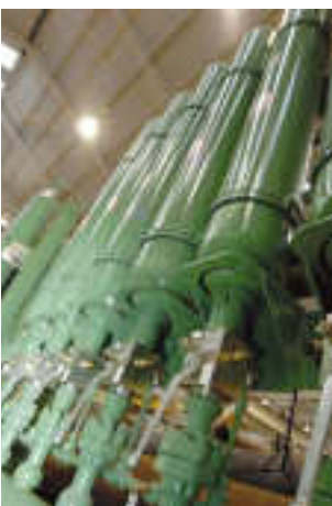
New power pack for cylinder forge - September 2005
